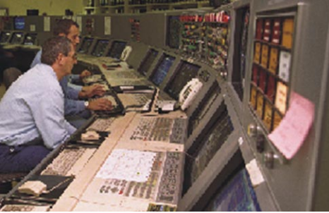
Effectively designed control rooms present control system data "at-a-glance"
