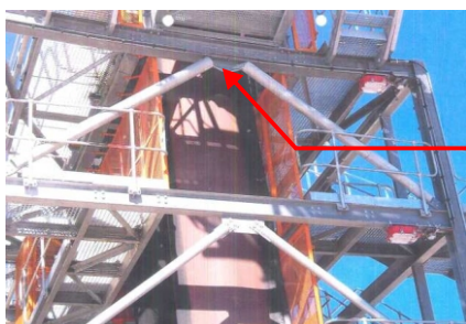
Buckled Light Bracing Due To Eccentric Connection
